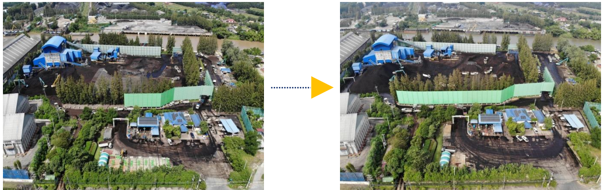
Pictures show the progress of a permanent wind break construction at the Coal Distribution Center, Phra Nakhon Si Ayutthaya Province
